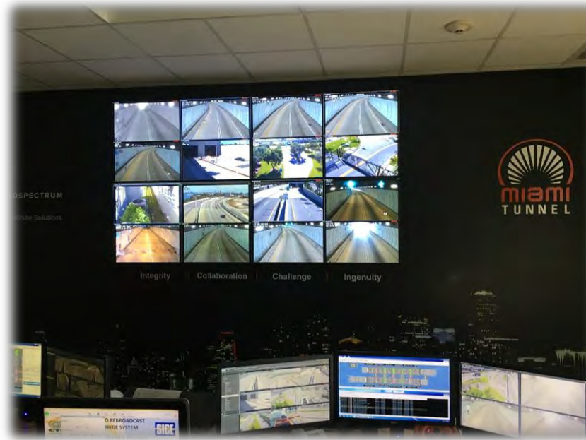
Traffic Management Center – Miami Tunnel to Port of Miami 2018
